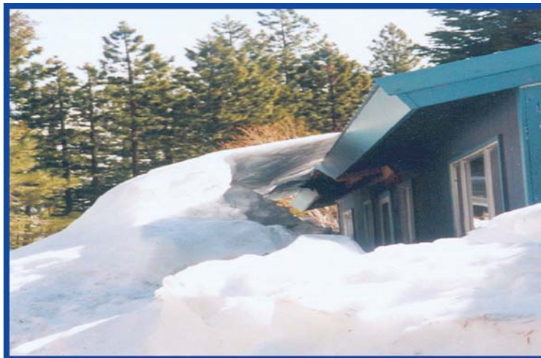
Photo 2: Dormers can be torn off.
